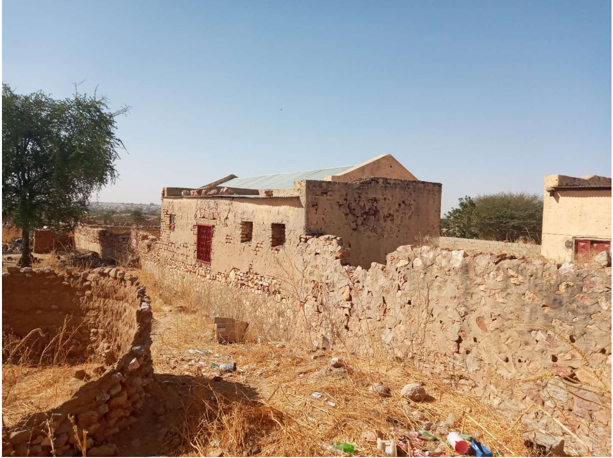
Figure 5. Part of the fence to be repaired
