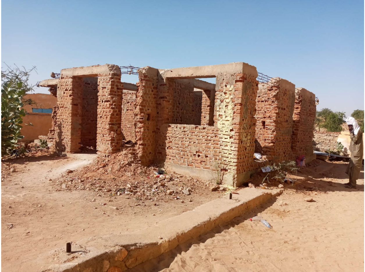
Figure 1. Existing building for Blood bank. To be demolished for a new construction
