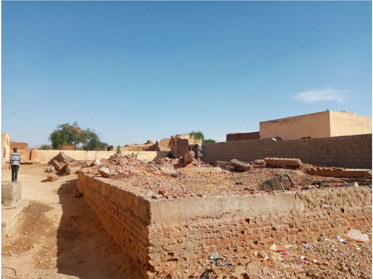
Figure 2. Existing foundation to be demolished for construction of wards as per building no.8
